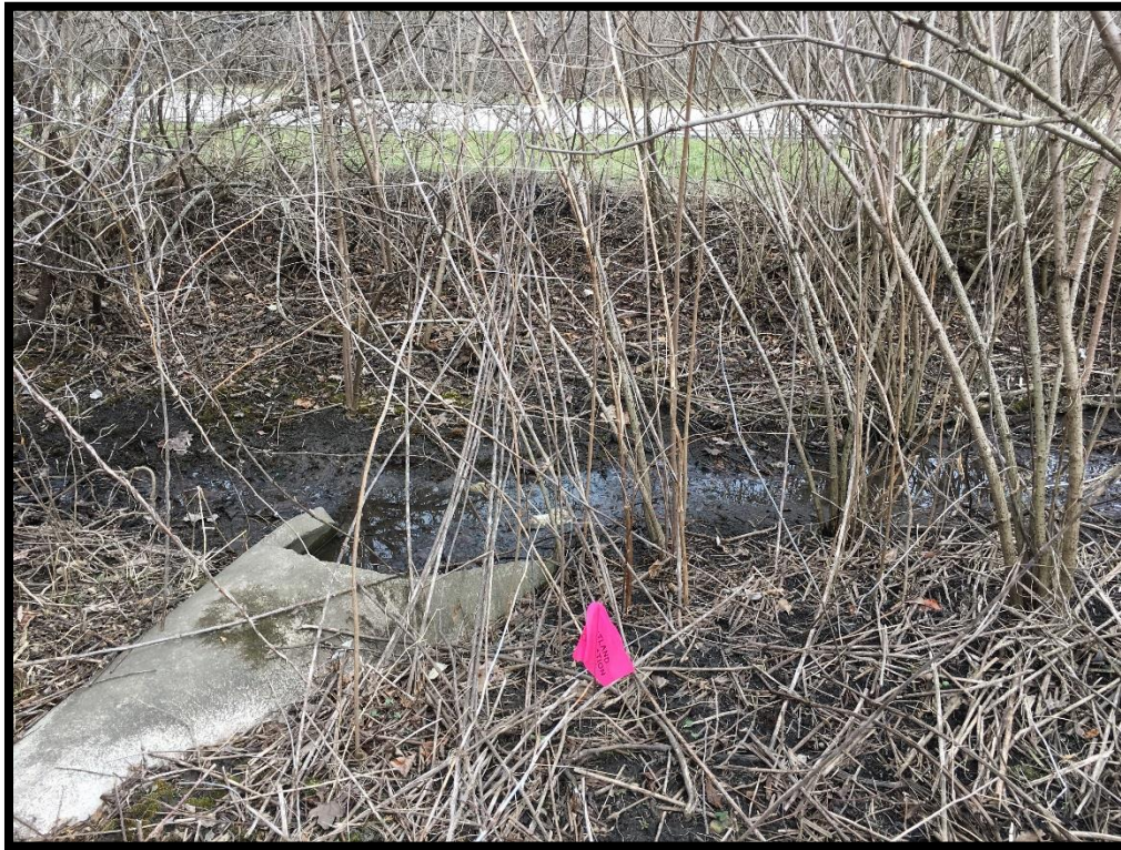
Pipe outfall at NE corner of lot near Kenosha Bike Path – facing east
